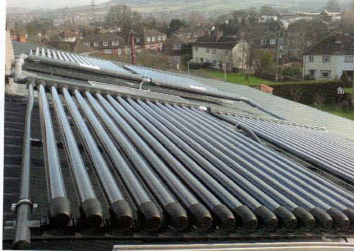
Solar thermal – using evacuated tube collectors extends harvests into the winter.
